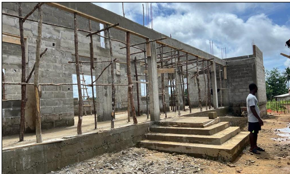
Figure 1: ECE School Construction Works at P.G. Neh, Gbanken; Grand Kru County - God Trust Construction Company
