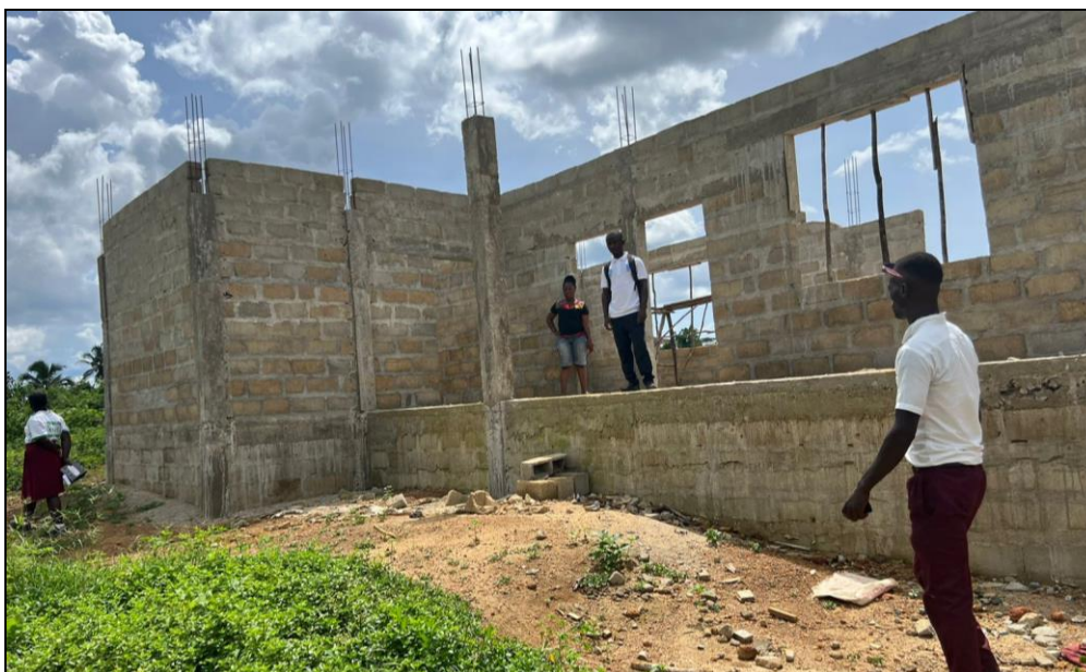
Figure 2: Ongoing ECE School Construction in Geetroh Togbaville in Sanquin District, Sinoe County being implemented by Classical Group of Companies.
